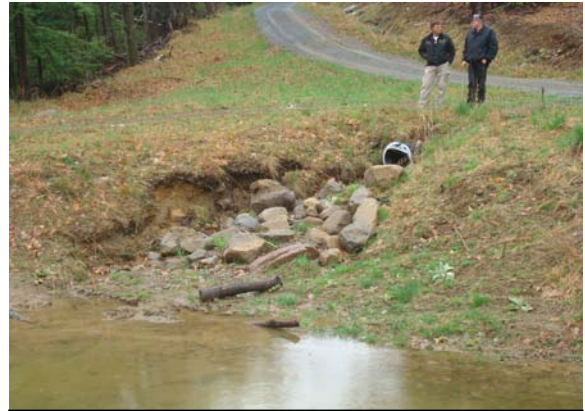
Inlet to a retention basin which needs to be re-shaped and stabilized. This basin is full and is in need of cleanout for it to function as designed.
