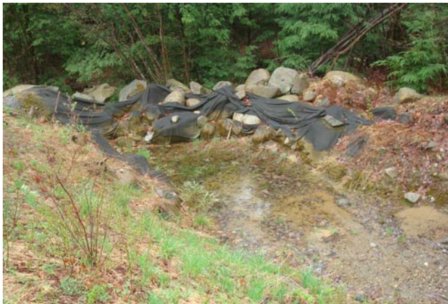
Retention pond in need of reshaping and stabilization.
