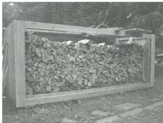
Keep firewood dry, off the ground, and stacked so air can circulate throughout the ranks. The roof on this firewood rack is being constructed.
